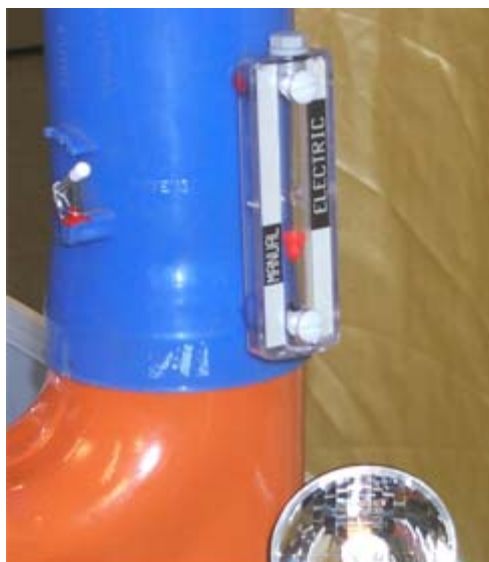
The air flow is monitored from an air flow meter indicating ranges for electric and manual blower operation. Note the incorporated emergency light
